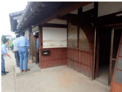
Damage to houses in Saga Prefecture (Takeo City) (Source: Cabinet Office)
