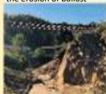
The Sanriku Railway, the erosion of ballast
