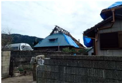
Damage to houses in Chiba Prefecture (Futtsu City) (Source: Cabinet Office)
