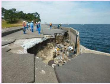
Damage to bank protection at Kanazawa District, Yokohama City
